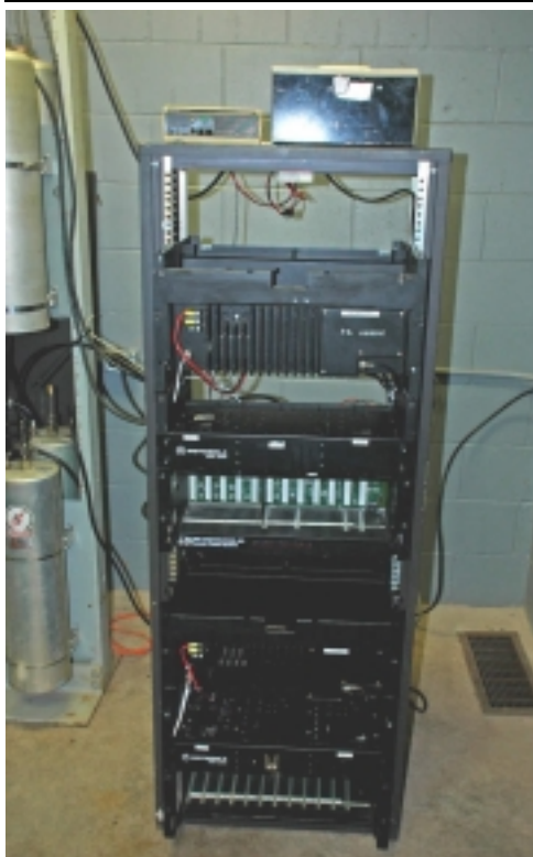
The VE1CFR MSR-2000 repeater duo with the UHF bottom, VHF top, RLC Controller in the center and GE Phoenix with power supply on top of the cabinet installed 2008-03-01 Photo taken by Ron VE1AIC.
